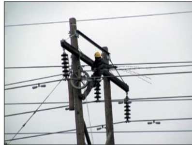
Fiber shares towers here with a high-tension power line.
