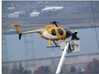
Much of the fiber in the The Dalles network is aerial. This construction shot gives an idea of the area's charm.
